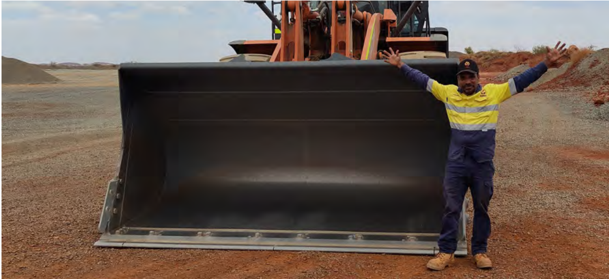
Terrance Warrie with his loader, while working on the Ventia/Main Roads project.
