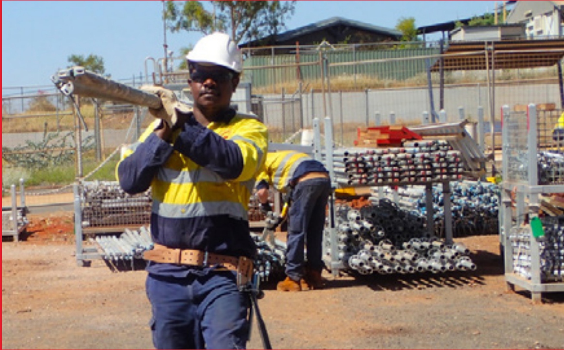
Yurra employee Curtis Lockyer while working on the Ganalili renovation. Photo: Yurra
