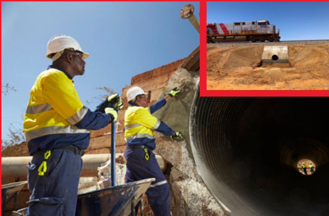
Local workers maintaining a rail culvert as part of Yurra's $20 million rail maintenance contract with Rio Tinto.
